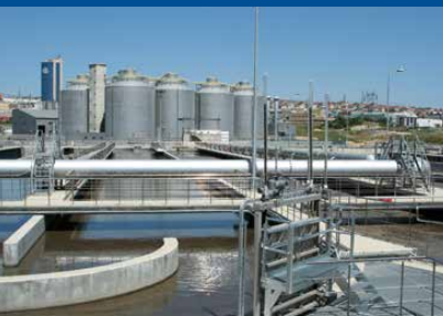
Activated Sludge Tanks and Digesters
