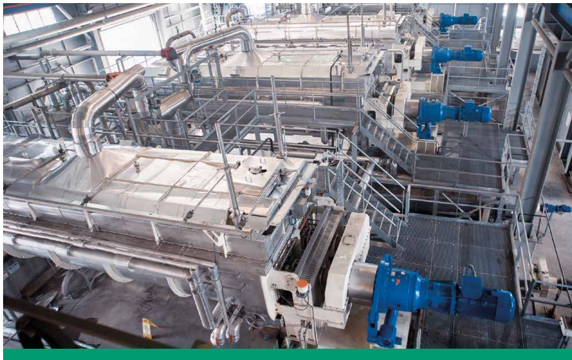
Sludge Drying Units
